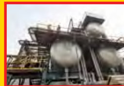
State of art lube oil blending plant built in Taloja
